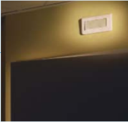
Illuminated bulkhead light on above the entrance to bathrooms.
