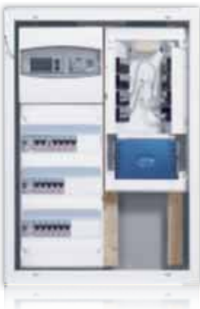
MULTIMEDIA DISTRIBUTION BOARD
