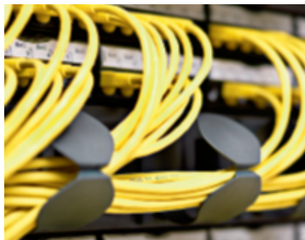
Patch panel (p. 90)
