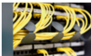
Management panels: with rings to guide and protect the patch cords.
